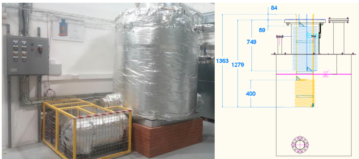
Figure 52. TESLAB tank (left) and drawing of the helical coil (right)
